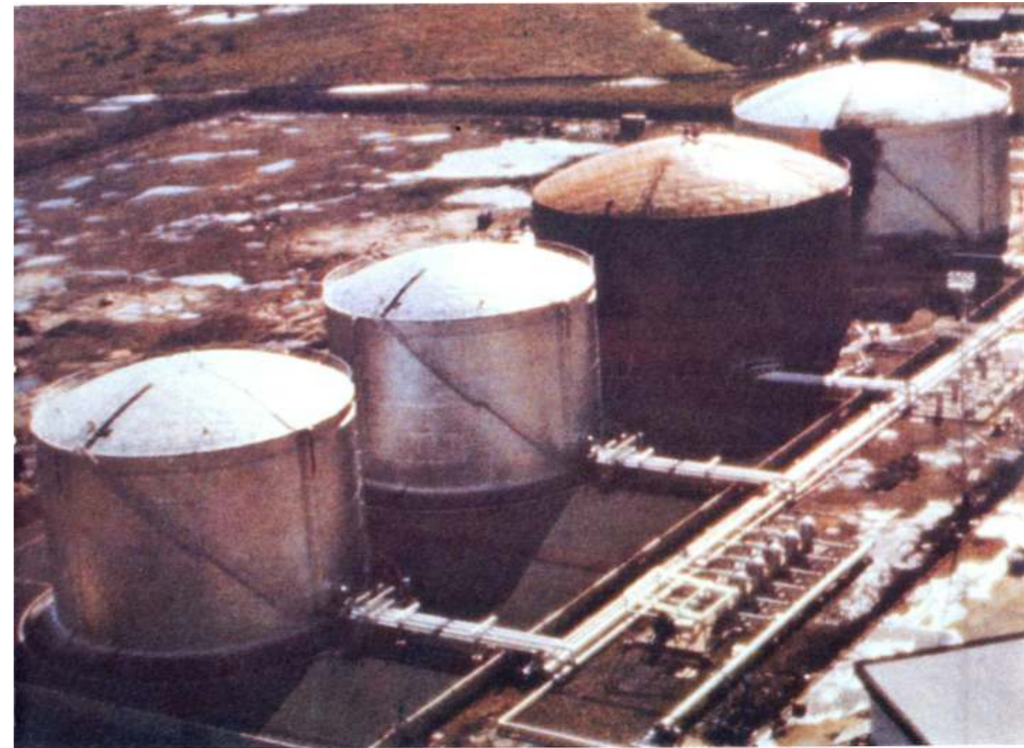
A turnkey Petroleum Storage and Handling Terminal executed for Kenya Pipeline Co. Ltd., Nairobi involving complete storage and pumping facilities along with all civil, electrical, instrumentation and piping work.
