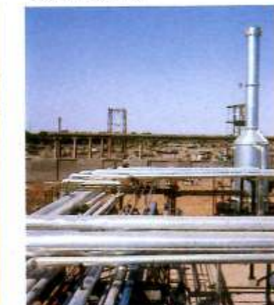
12 Crude Distillation unit IOC Gujarat Refinery
