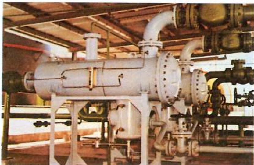
Filter Water Separators as part of a Aviation Fuelling Facility provided by VTV at Hulule, Maldives.
