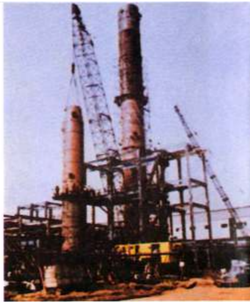
Site assembly at RCF, Bombay of a VTV shop fabricated Benfield Regenerator and Benfield Absorber.
