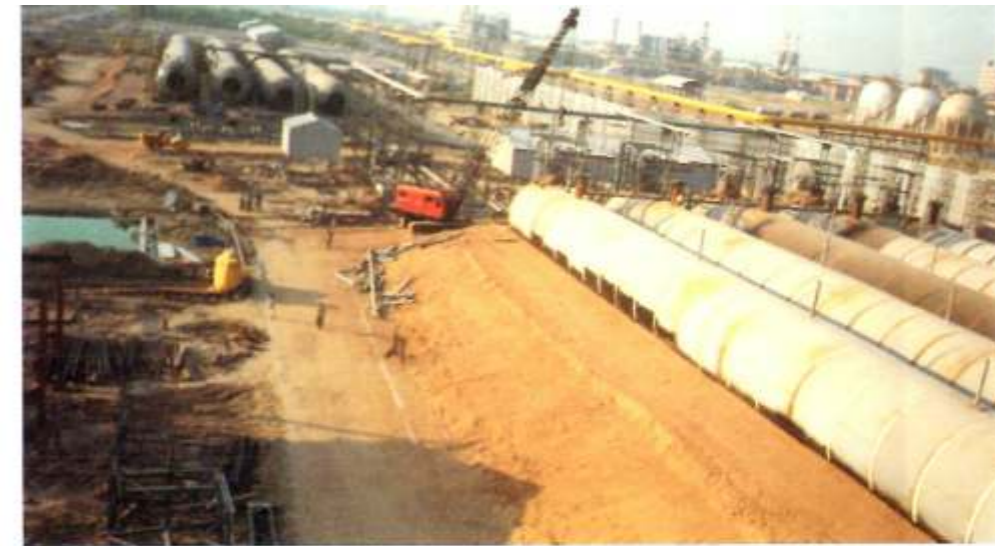
India's largest LPG mounded storage terminal designed, constructed and commissioned by VTV for The Gas Authority of India Ltd., Patna.
