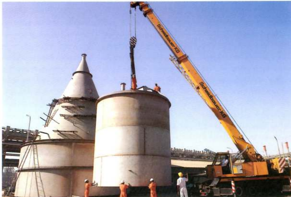
Stainless Steel Silo subassemblies under final erection at a petrochemical complex. VTV's diversified product portfolio enables it to provide single point responsibility for a wide range of services on large industrial projects.
