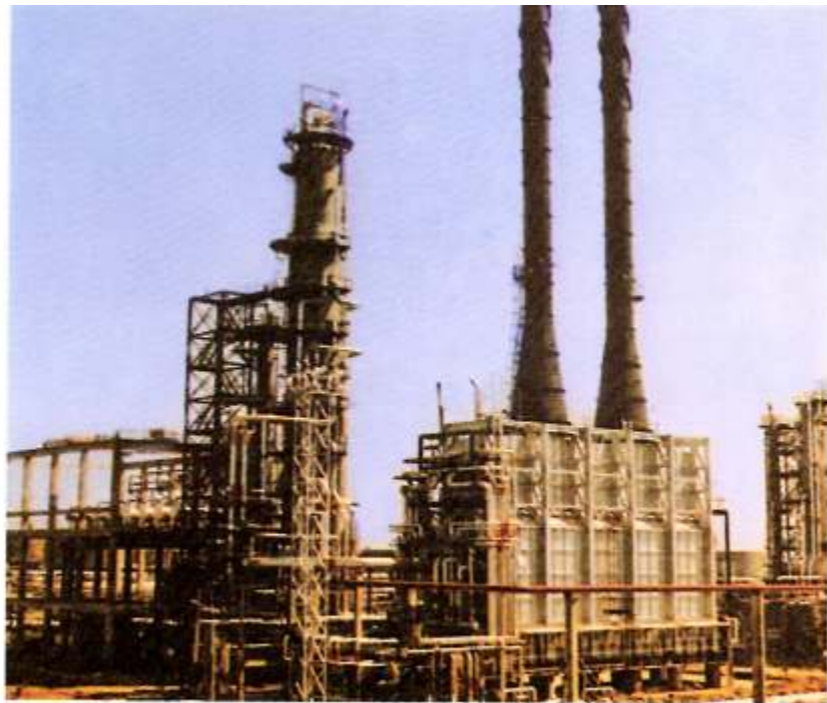
A Crude Distillation Unit constructed by VTV for a 12mtpa Oil Refinery in Gujarat.
