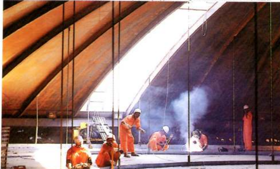
The outer tank dome roof and suspended deck of a cryogenic propylene storage tank constructed for RIL, Hazira.
