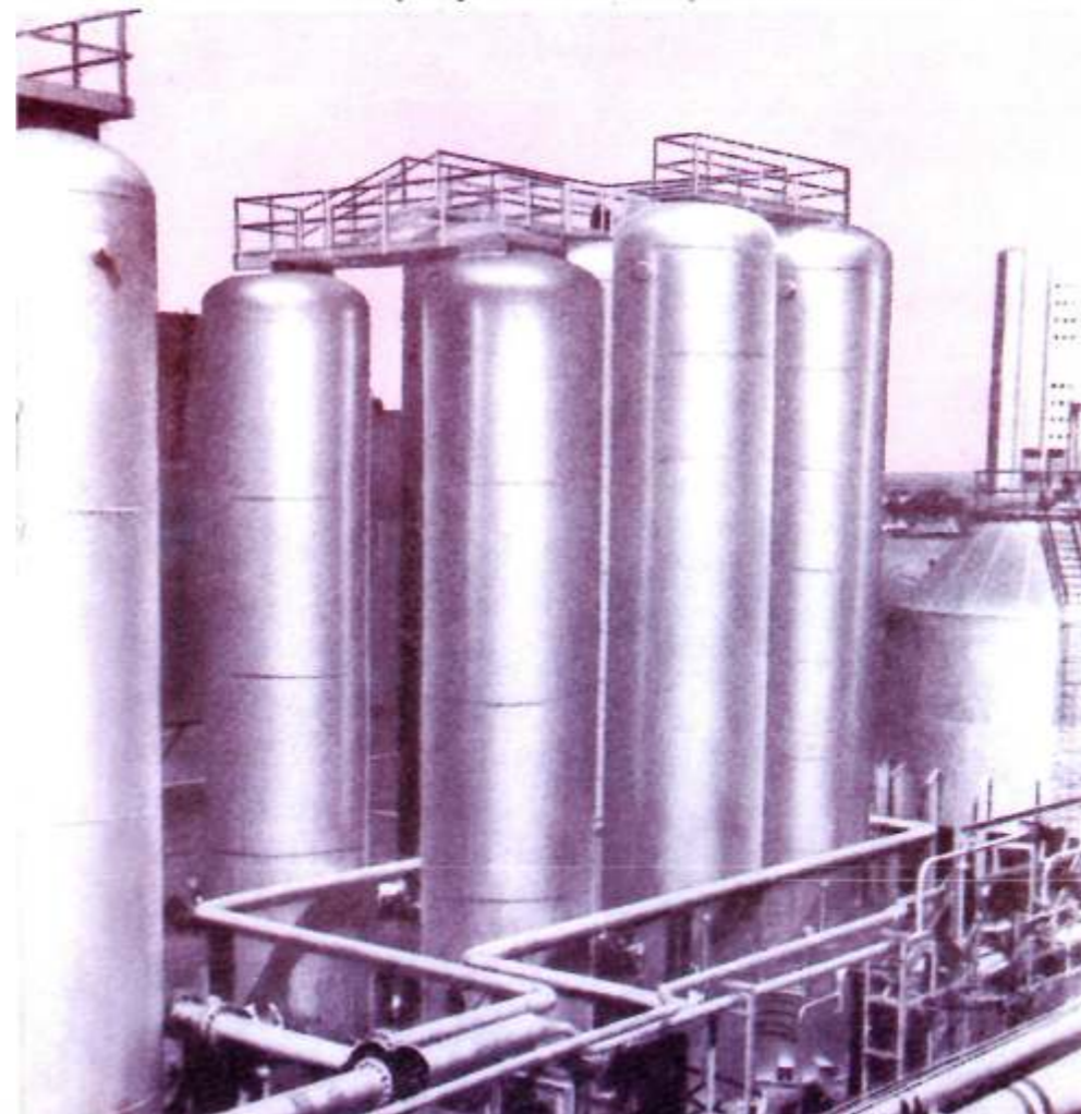
Gaseous Oxygen Vessels provided as part of a turnkey cryogenic storage and handling facility designed and constructed by VTV for Bilhat Steel Plant.
