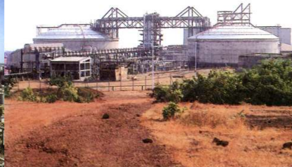
VTV pioneered the EPC execution of 9% Nickel Tanks in India with a 23000 Mt. cryogenic storage terminal for IPCL's Nagothane Petrochemical Complex.
