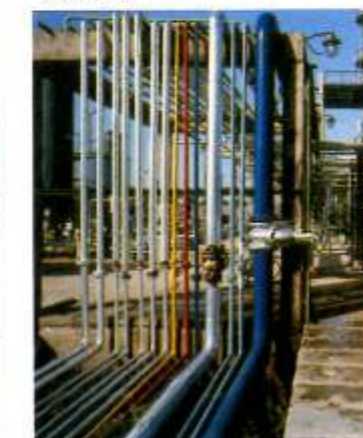
8 Process Piping Sangamner Refinery & Petrochemical Ltd.
