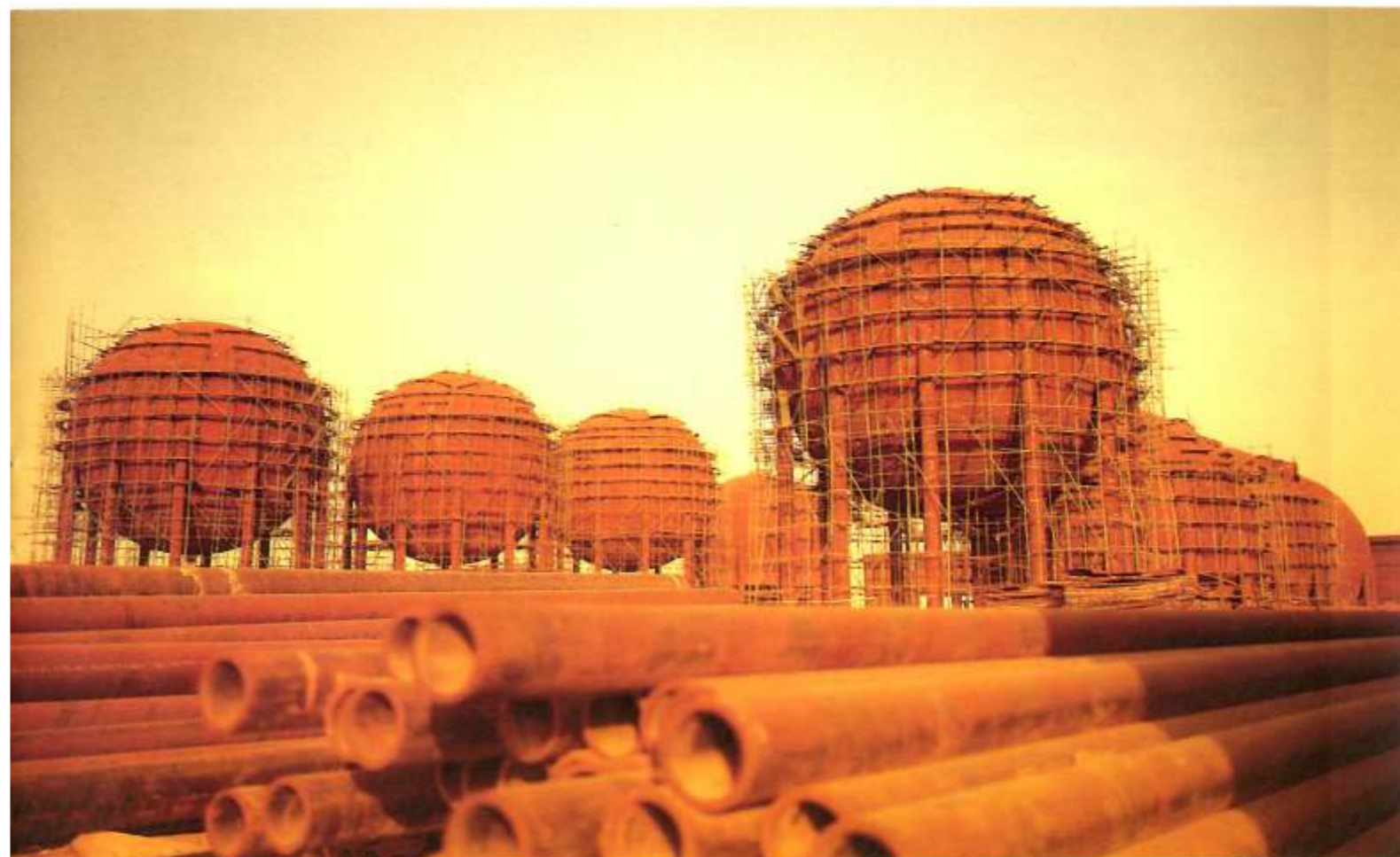
A 23000 cu.m. LPG storage terminal, amongst India's largest, designed and constructed for Essar Oil's Jamnagar Refinery.
