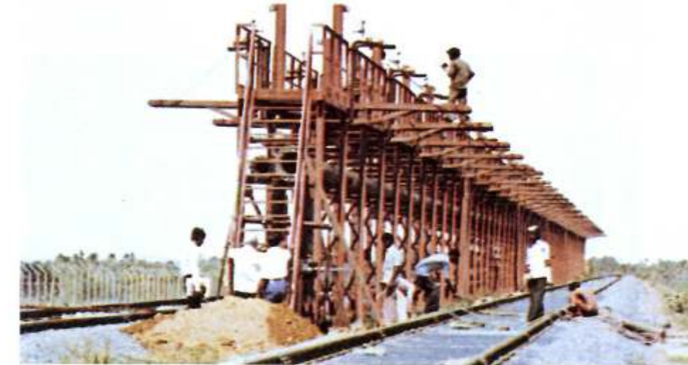
A 60 LPG tank wagon unloading gantry designed and constructed as part of a turnkey LPG storage and handling facility delivered by VTV to Salem Steel Plant.
