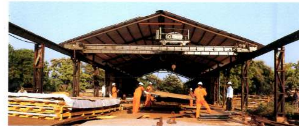
A covered mobile fabrication gantry temporarily installed by VTV at the worksite for handling 9% Nickel Steel prefabrication of 4 nos. ethylene cryogenic storage tanks for Finolex, Ratnagiri.
