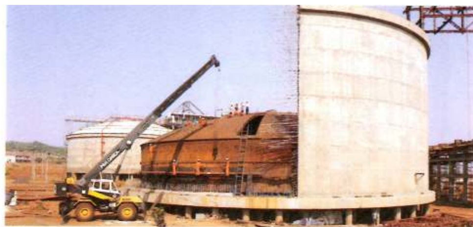
After completion of the outer tank top shell course, dome roof and suspended deck of this 9% Nickel Tank, hydraulic jacks were used to progressively lift and construct the tank to its final position with all work being handled at grade level.
