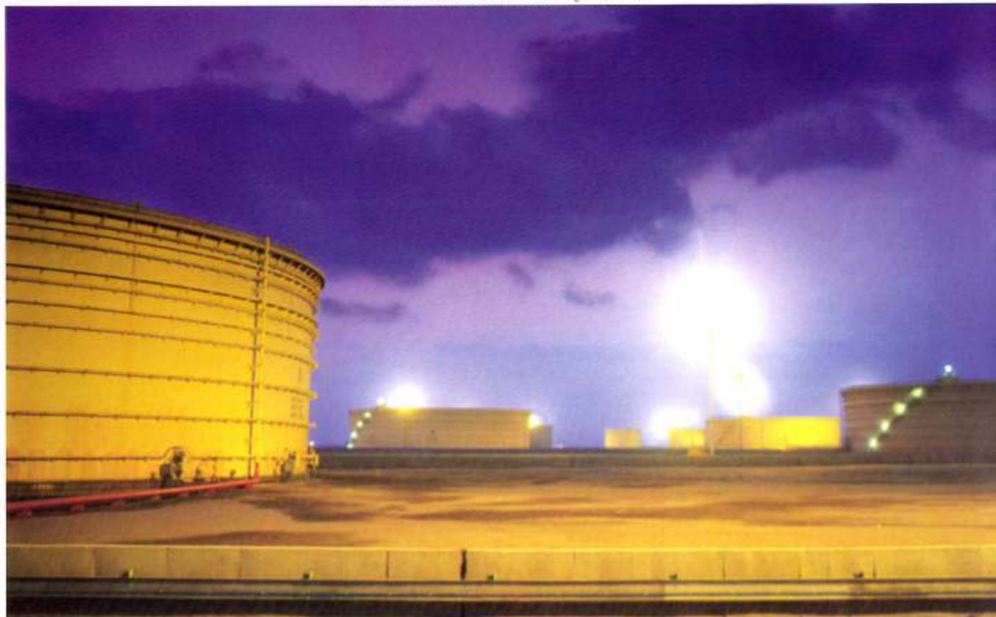
A global scale crude oil tankfarm designed and constructed by VTV for RPL's Jamnagar Refinery comprising of 12 nos. 92 m dia. X 20 m ht. double deck floating roof tanks.
