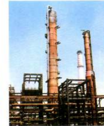
5 Vacuum Columns BPCL Mumbai
