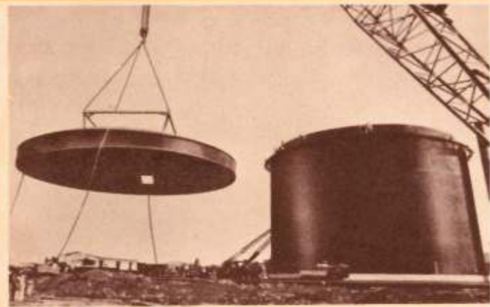
3,000 metric tonne double integrity ammonia storage tank being fabricated at Sri Lanka
