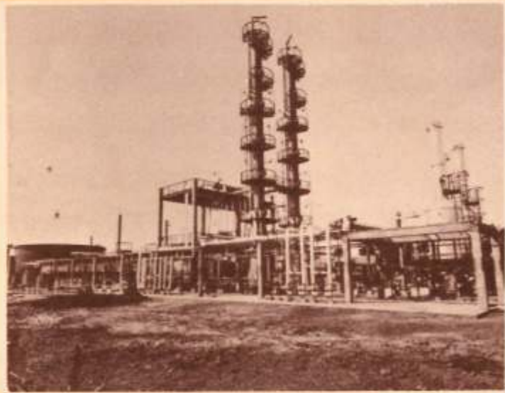
Pilot distillation facilities for Gujarat Refinery to process feedstocks for producing special products
