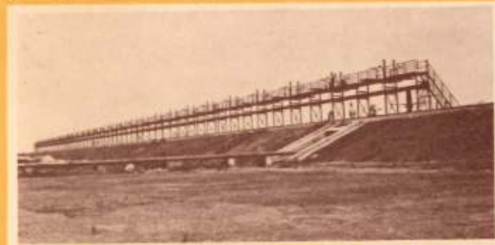
A 60 LPG tank wagon unloading gantry for Salem Steel Plant
