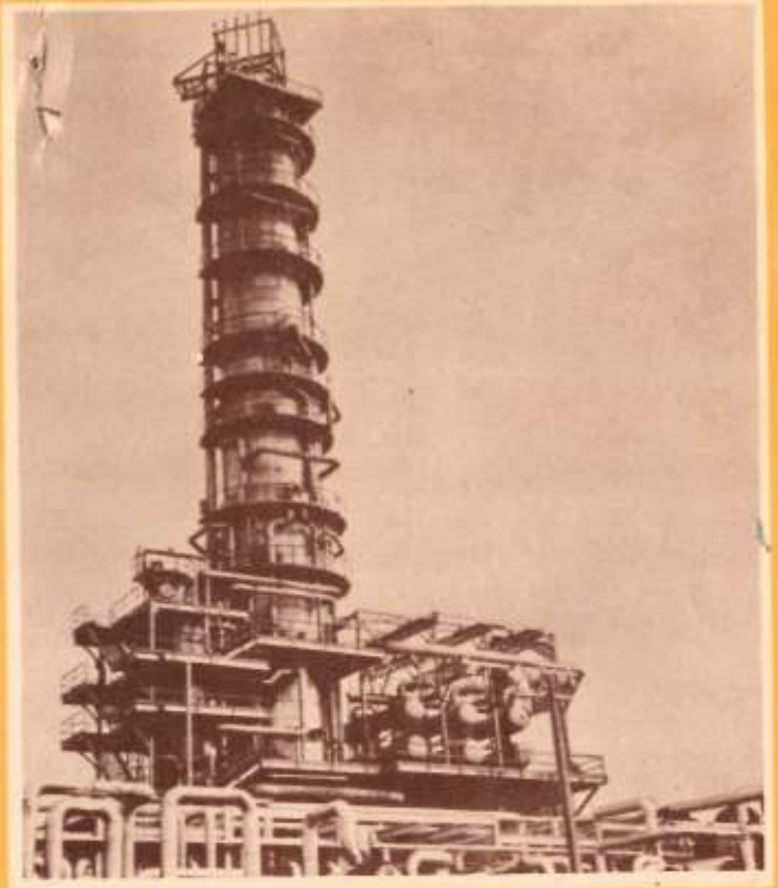
5 m dia x 52 m high crude distillation column at Hindustan Petroleum Refinery
