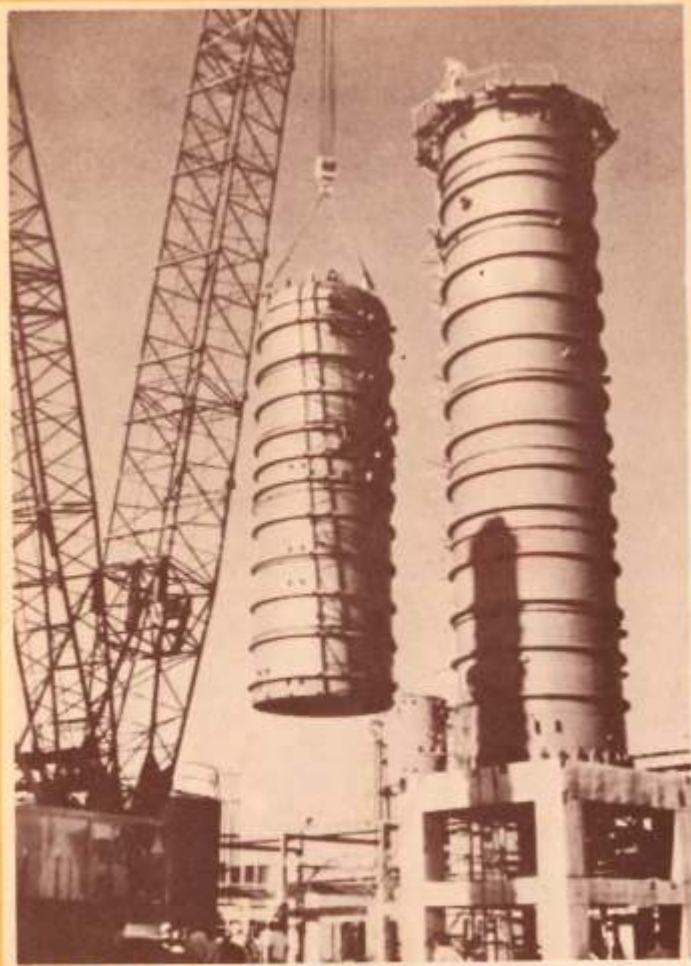
A 4.75 m dia x 40 m high fractionating column under final assembly at a Petrochemical Complex
