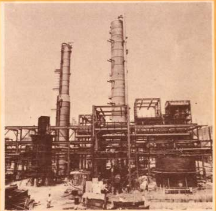
The various stages of site assembly of shop fabricated Benfield Regenerator and Benfield Absorber
